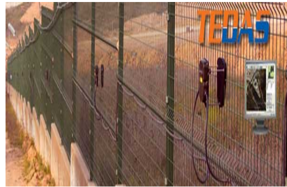
Fig.1 TEDAS Sensor Network System for Intrusion Detection
